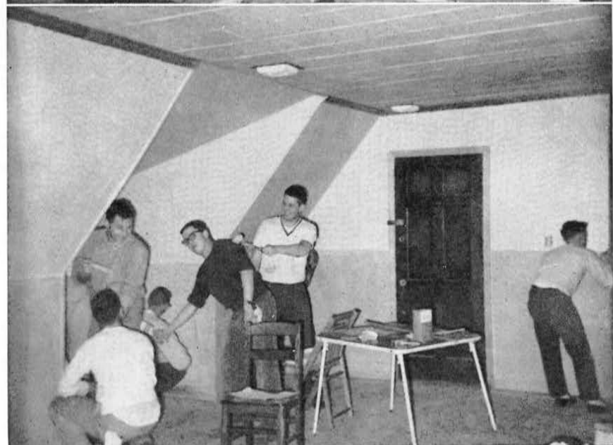
Iotans are at work on the recreation room. From left to right, you see Ernest Jones, Bill Dausch, and John Squire. Below: Jerry Greetham, Ted Schobert, Earl Veits, John Rapack, and Lee Coppess are at work on the temporary pledge room which will be made into study rooms in the Ohio State house
